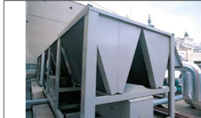
EQUIPAMIENTO PRINCIPAL: 2 x EUWA200MZ
